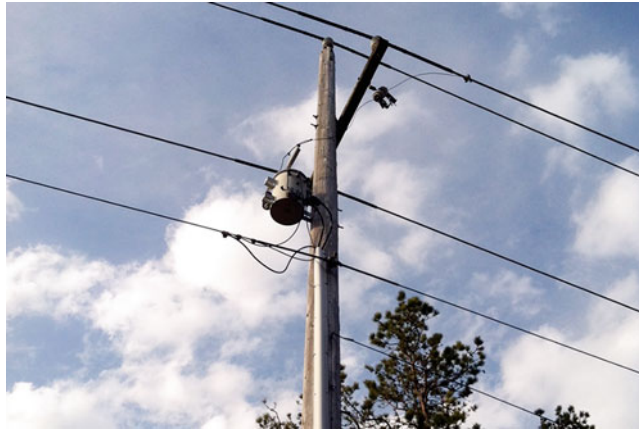
Fig. 11.18. Three-phase to three-wire residential system connected via a step-down transformer. From the pole transformer, the residential power system serving two houses is run down the pole underground. Cape Cod, MA.
