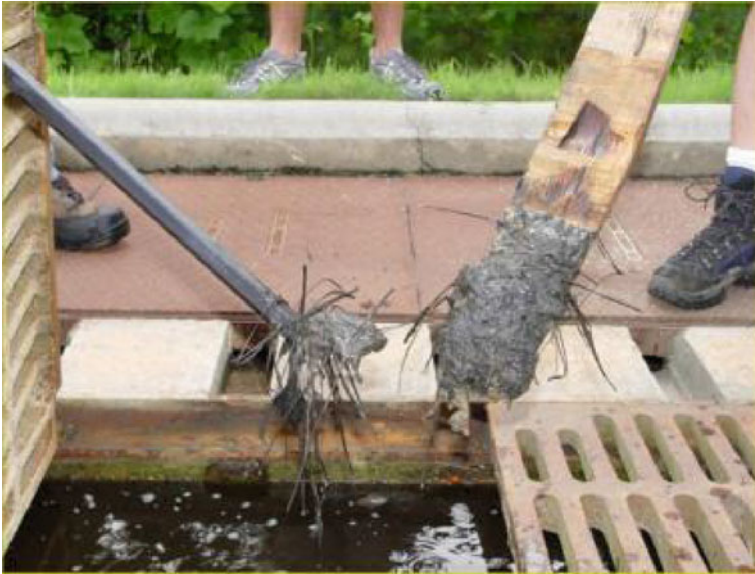
Gross solid accumulation in the sedimentation chamber
