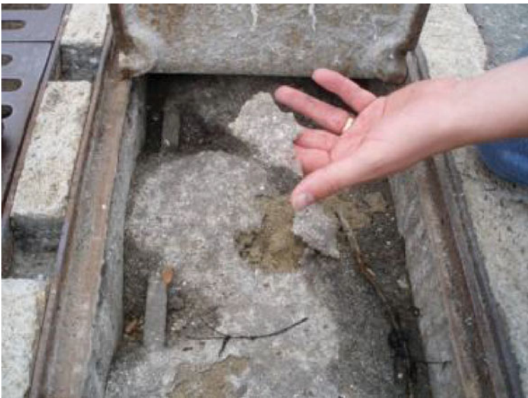
A smutzdecke (or polluted fines layer) in the sand chamber.
