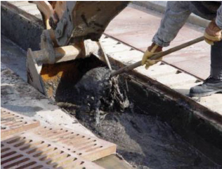
Shoveling accumulated gross solids and sediment into the bucket of a backhoe.
